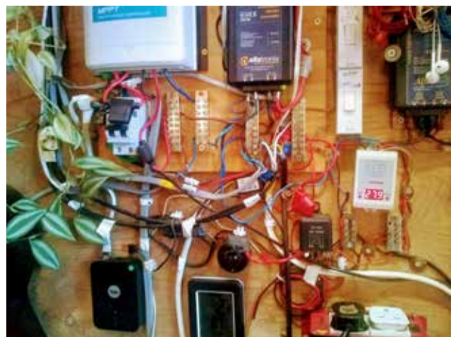
The 'electronic epicentre' of Hannah's off-grid system
